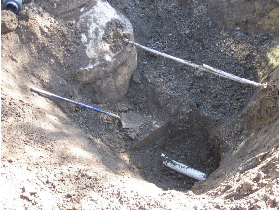
Photo 3: Condensate line exposed.
