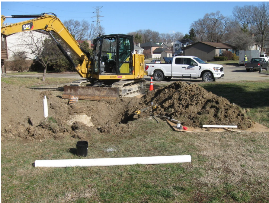
Photo 8: 4-inch ID PVC riser and 1 ½ inch ID PVC valve stem in place.
