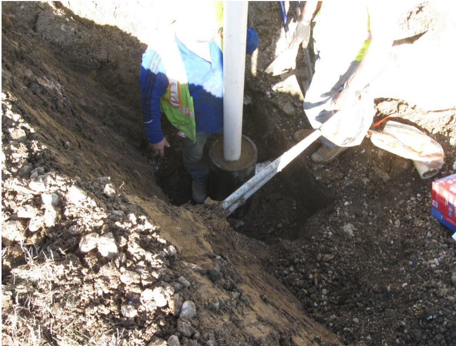
Photo 7: 4-inch PVC riser placed above valve. Annulus between 10-inch ID HDPE sleeve and 4-inch ID PVC riser filled with sand.
