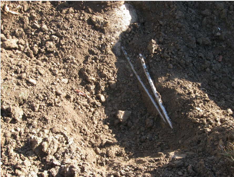
Photo 2: Conduit for high level alarm exposed. Note that a scrap piece of conduit was placed in trench.
