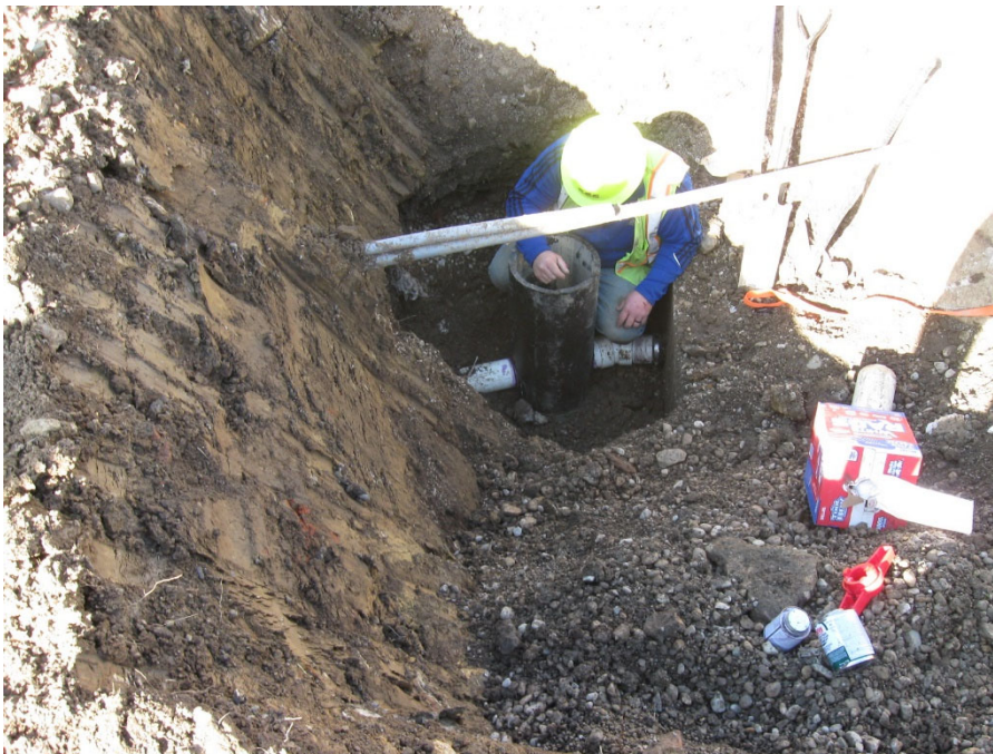
Photo 6: 10-inch ID sleeve of HDPE pipe placed over the valve.
